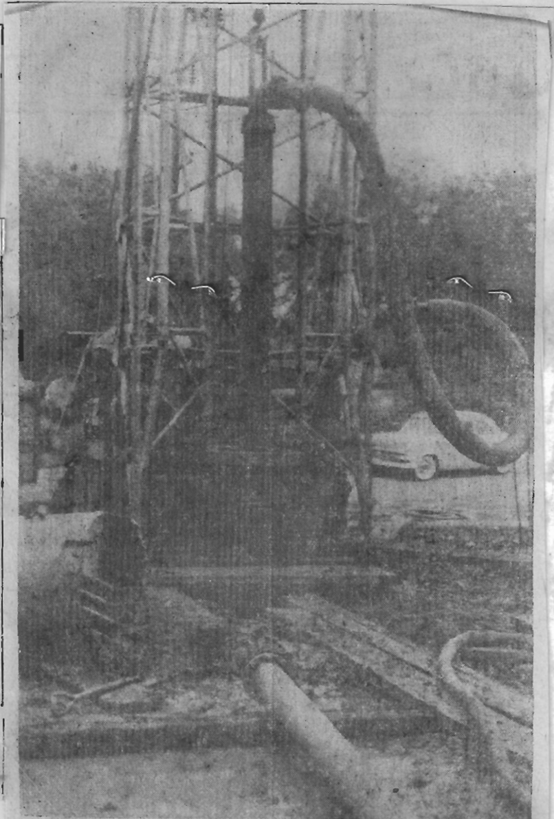
DRILL POUNDS DEEPER —Dick Kunkle and Guy Lemar, both of Stewart, Ia., were drill operators when this picture was taken at the site of the new city water well. Drillers have been averaging about 30-feet per day with 2,700 depth foot as the goal.
