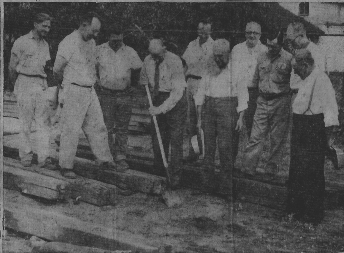
CIVIC MILESTONE — Councilman George Clifton, chairman of the water committee, shovels the first dirt Friday in ground-breaking for the city's new deep well as other council members and the mayor await their turns. In the group, left to right: Bernie Matherly, waterworks superintendent; Councilman Bob Breiting; Don Kunkel, driller for Thorpe Well Co.; Clifton; City Engineer Don Ferguson; Councilmen Howard Sage, Carl Speth, John Hotchkin and Ed Speth; and Mayor Tom Godfrey.
