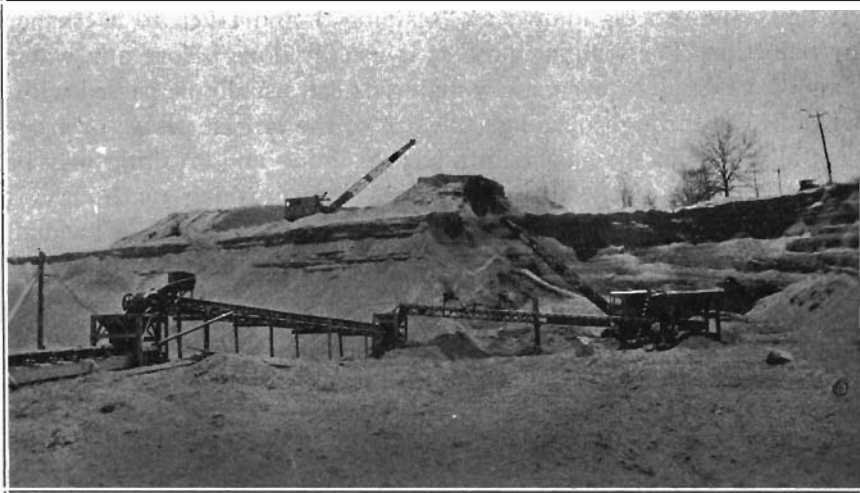
FIG. 29. — Bellevue Sand and Gravel Co., Bellevue. View of the Belt Conveyor System.
